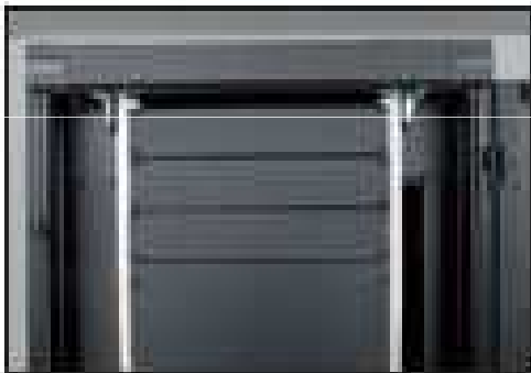
Side skirts and blanking panels
